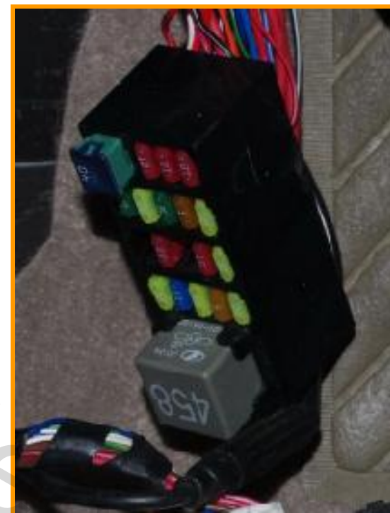
Instrument fuse box
