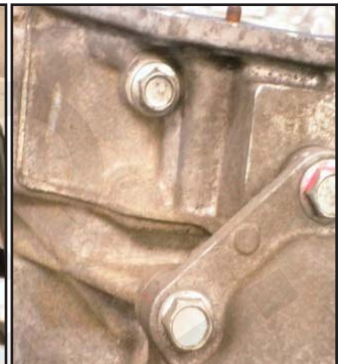
Outside pump bolt
